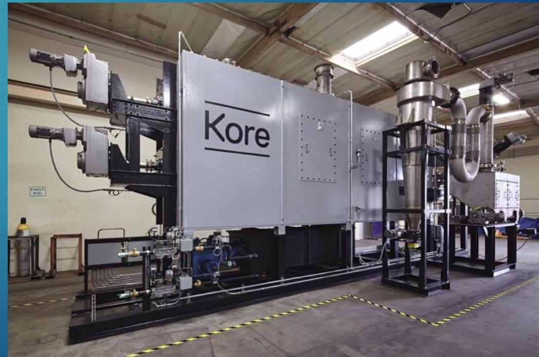
KORE Pyrolyzers for the Rialto facility
