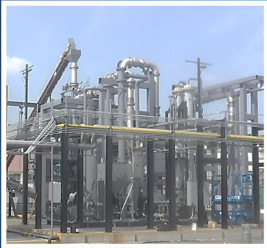
Pyro Gas conveyance and processing
