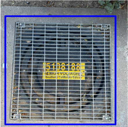
New Below Grade Electrical Transformer (Blue)
