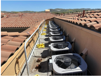
New Heat Pump Condensers with Fire Rated Shafts
