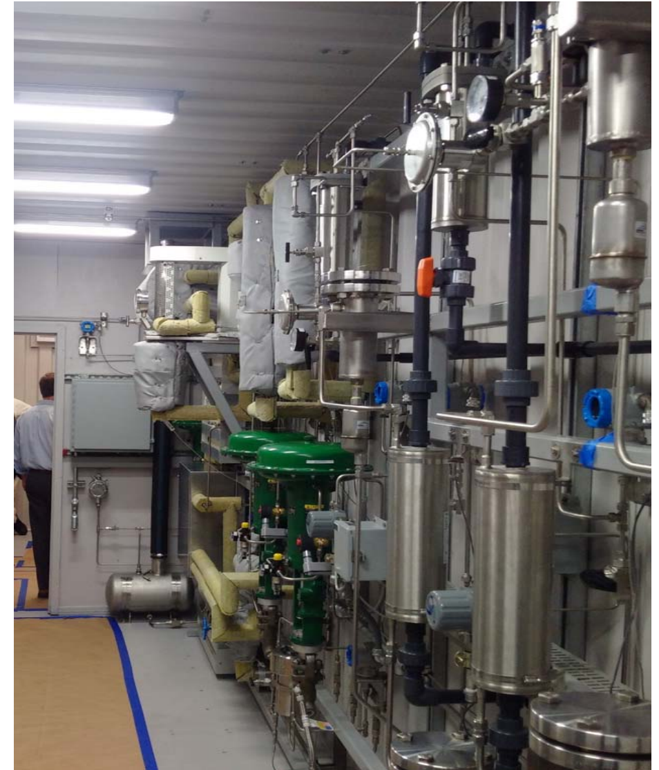
Genifuel dairy waste processing demonstration
