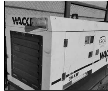
Portable Generators ≥ 50 BHP, Permitted/Registered w/ BACT for PM Emissions
