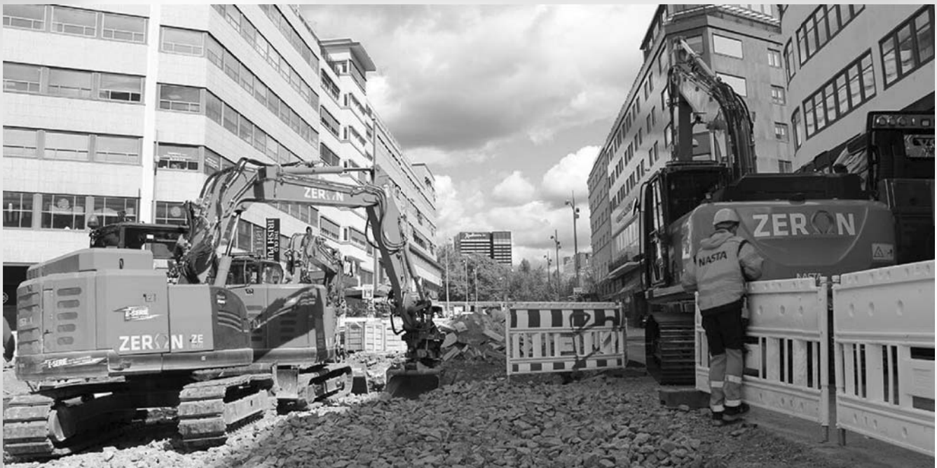
The Olav Vs Gate construction site in Oslo, Norway, is a zero-emissions project with ZERON ZE85US (9t) and ZE160LC (17.5t) electrified excavators built by NASTA AS. Courtesy of NASTA AS
