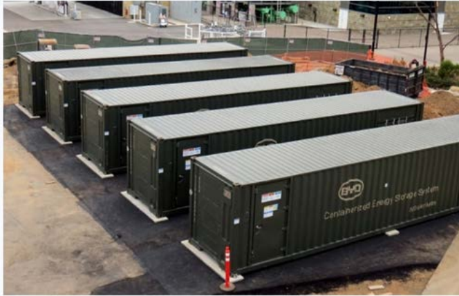
FIGURE 10-24 5 MW GRID LEVEL BATTERY STORAGE USED ON UC SAN DIEGO MICROGRID
