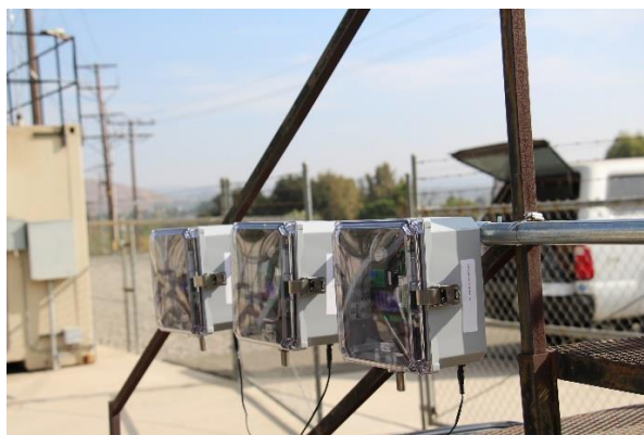
Figure 1.2. Co-location set-up for CSAM units #408 - #410 at Riverside-Rubidoux AMS
