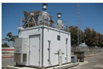
Fixed Station for Continuous Monitoring
