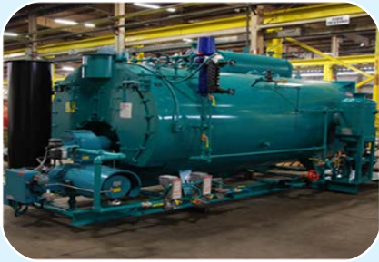
Boilers and heaters
