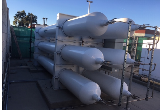
Figure 1: CNG “Cascading” Storage Tanks
