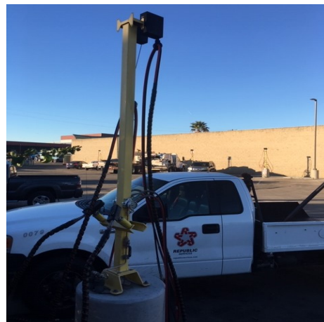
Figure 3: CNG Time-Fill Dispenser
