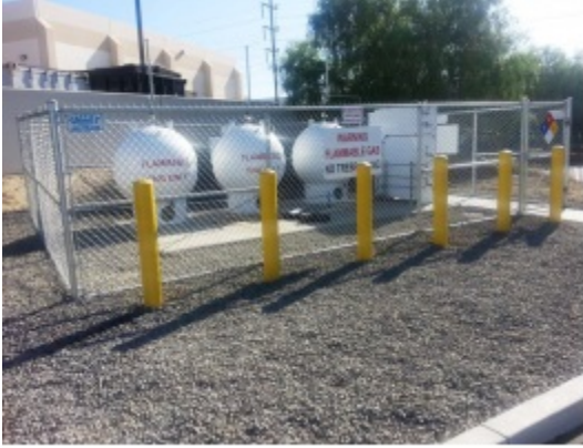
Figure 2: CNG Storage Vessels
