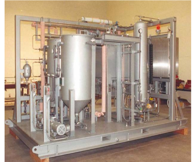
Skid-mounted HTP system
